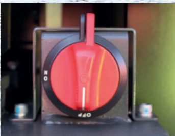
Battery cut-off switch
